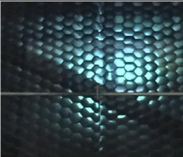
Lamella tubes after cleaning with air scour (Photos courtesy of Lee Schmidt, Manager of Water & Wastwater,
