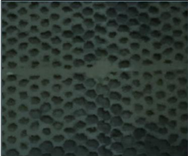
Lamella tubes after two weeks of operation
