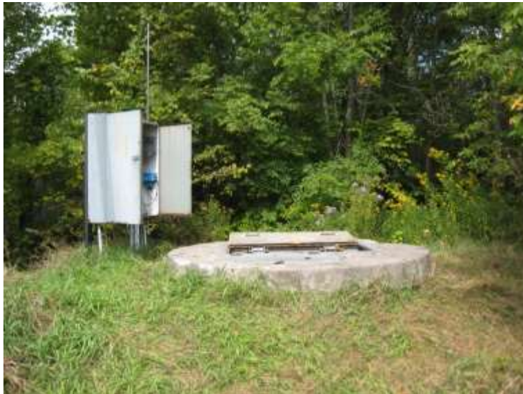
Underground Pumping Station
