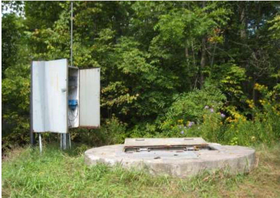
Lakefield College School Pumping Station Access
