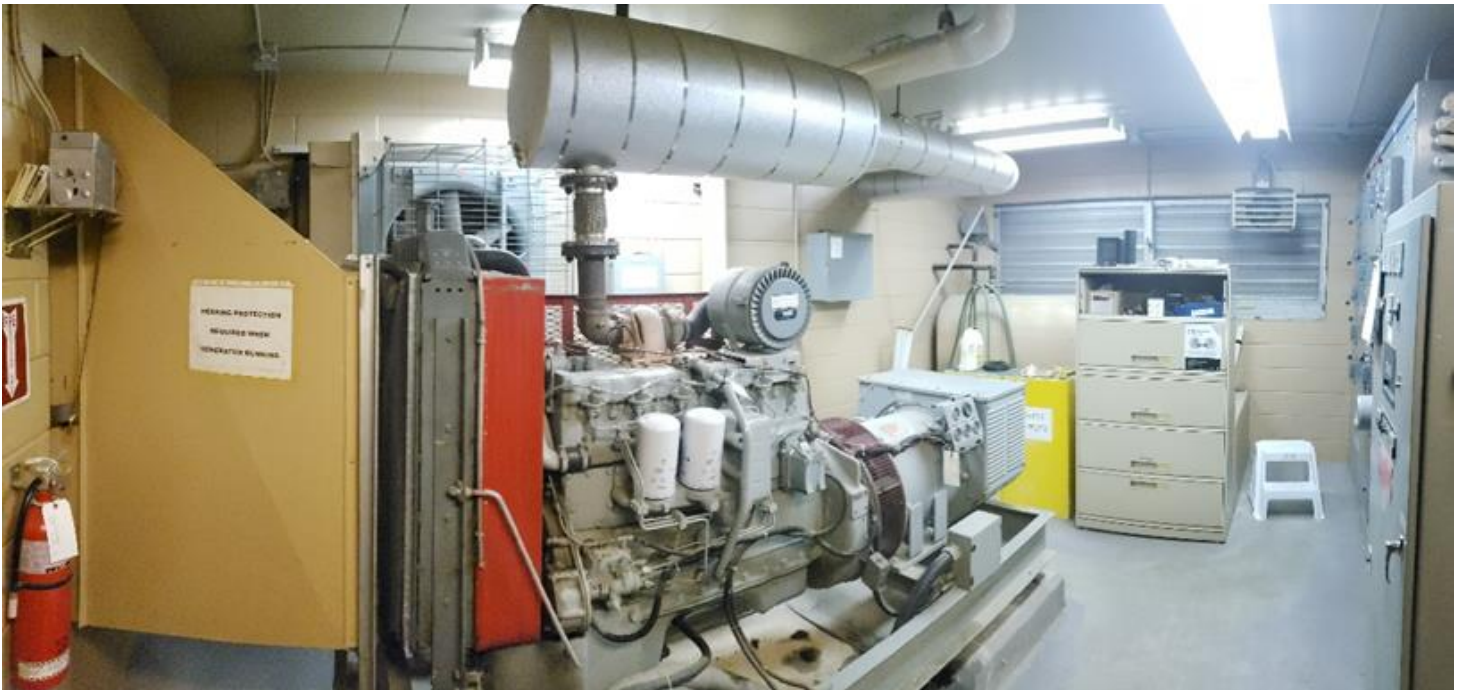
Existing 125 kW Water Street SPS Generator
