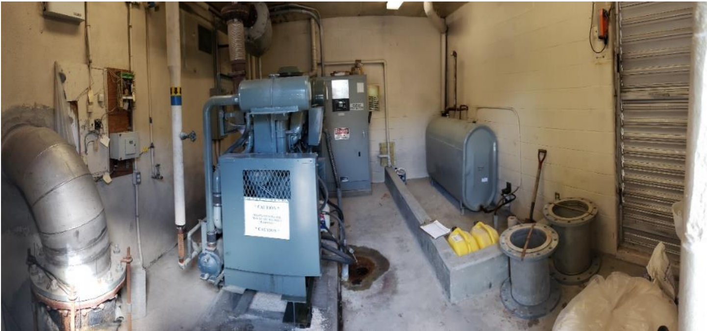
Existing Water Treatment Plant Generator System
