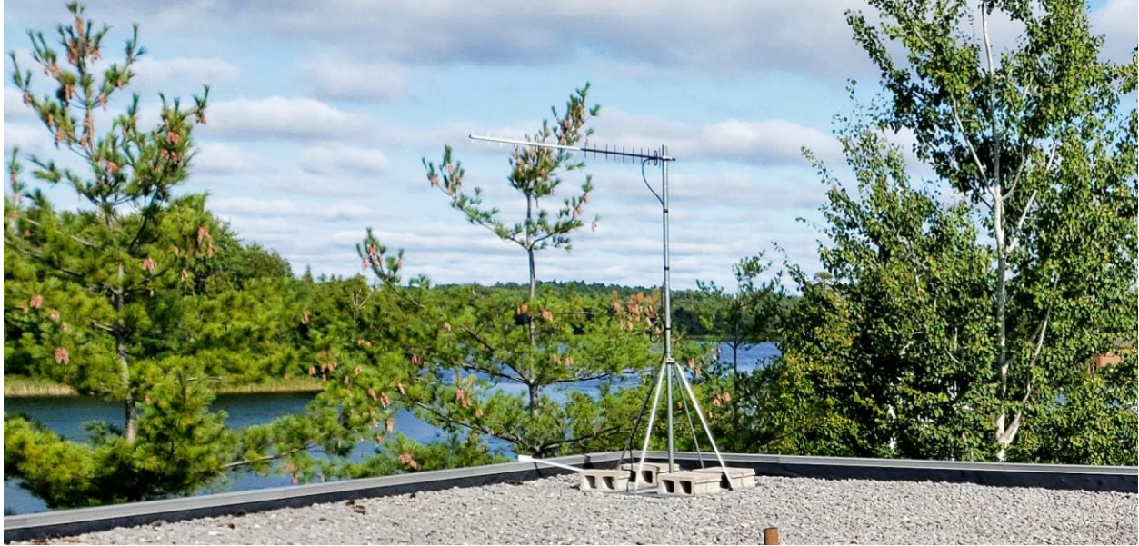
Existing WTP Radio Antenna and Mast
