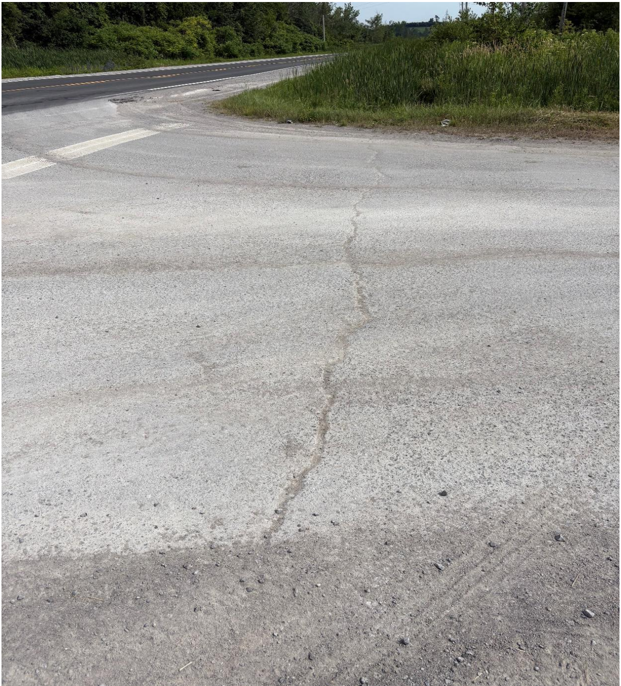
Photograph 1: Moderate Transverse Cracking (July 8, 2025)
