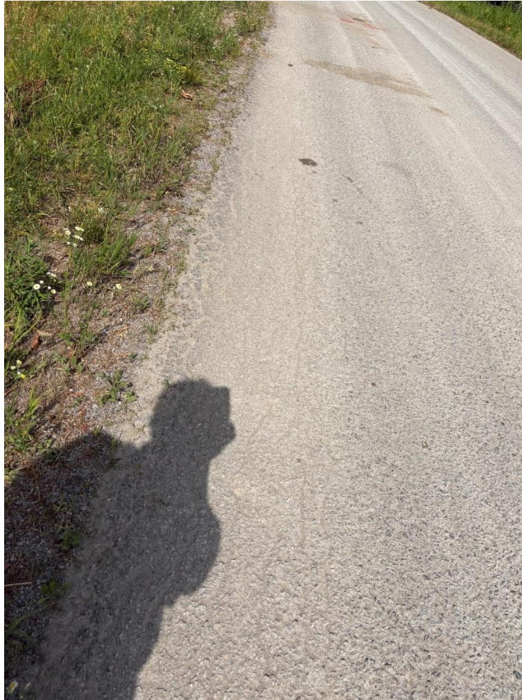
Photograph 6: Slight Pavement Edge Cracking (July 8, 2025)
