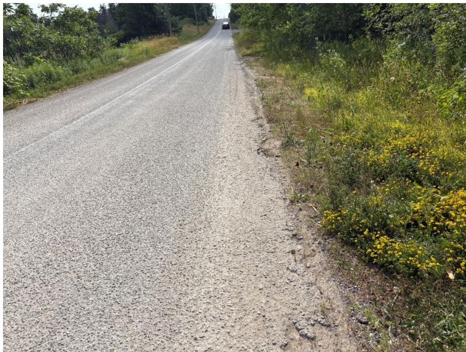
Photograph 7: Slight to moderate Pavement Edge Break (July 8, 2025)
