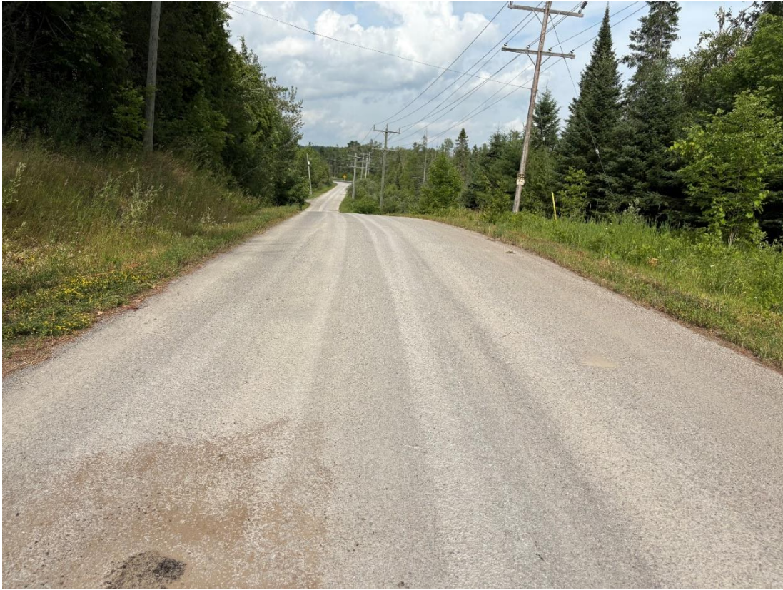
Photograph 4: Slight to moderate Wheel Track Rutting (July 8, 2025)
