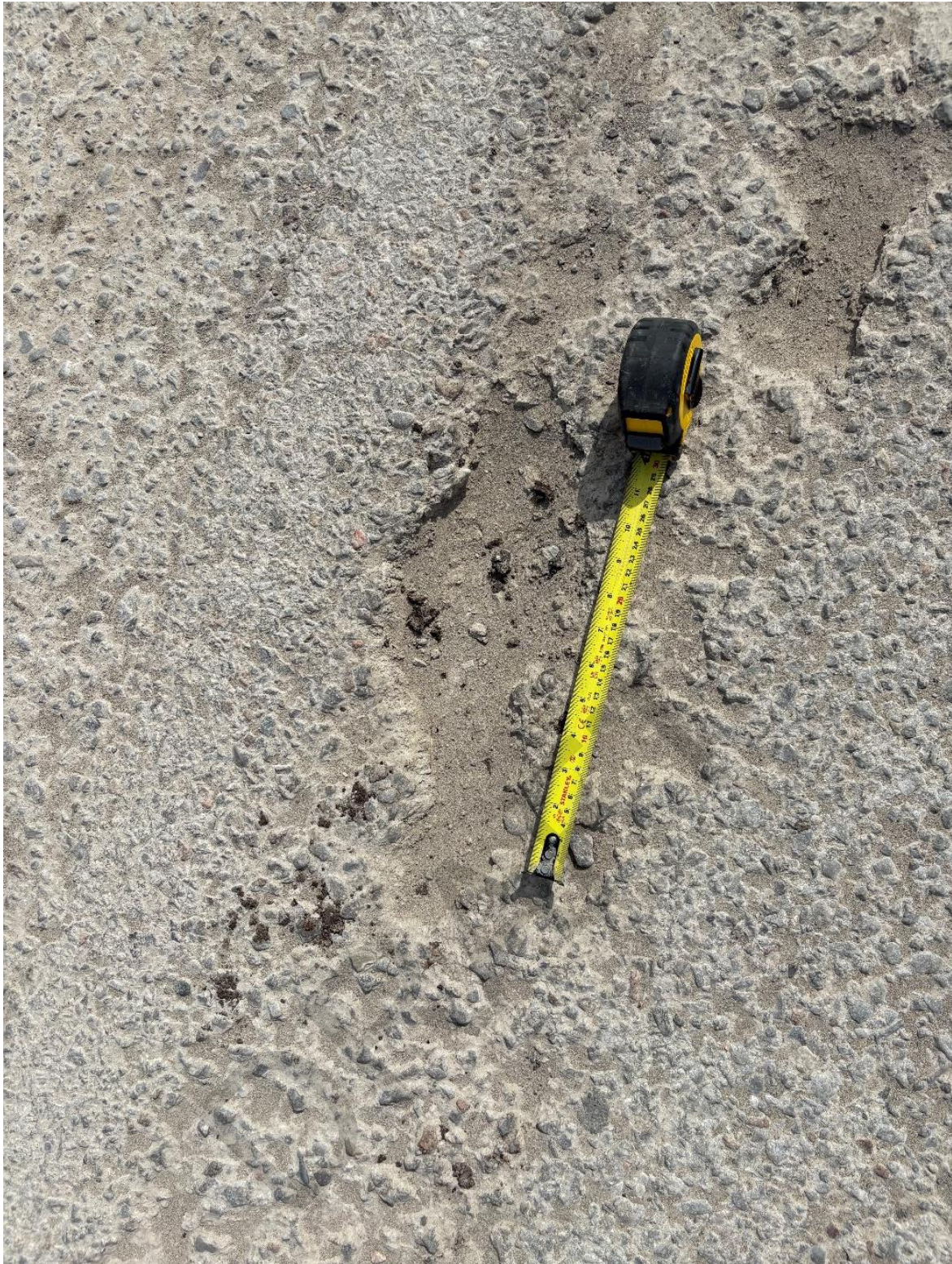
Photograph 3: Severe Ravelling (July 8, 2025)
