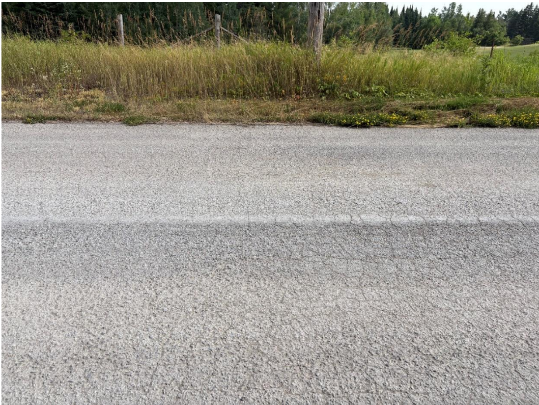
Photograph 5: Moderate Wheel Track Rutting and Alligator Cracking (July 8, 2025)
